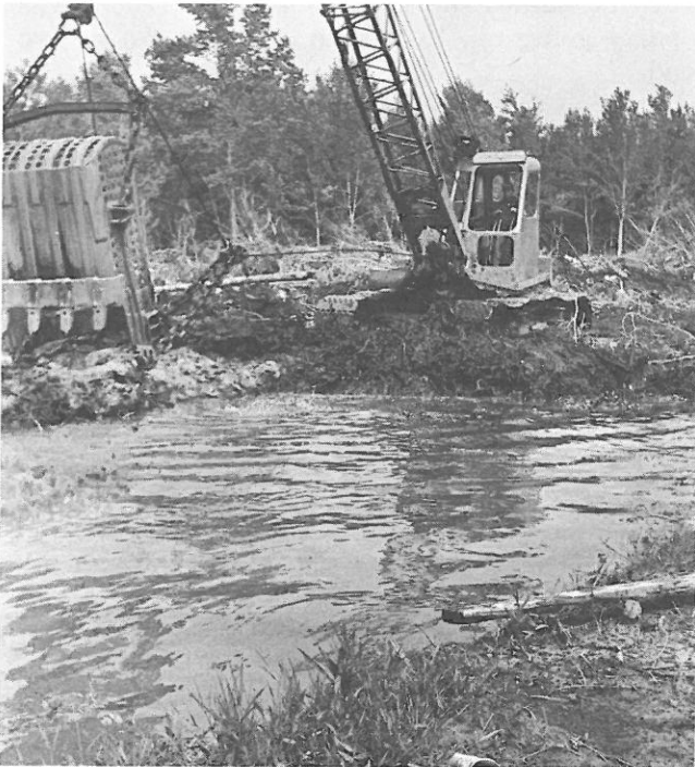
A dredging operation in the Rose Bay area. The water will eventually wind its way to Rose Bay itself.
