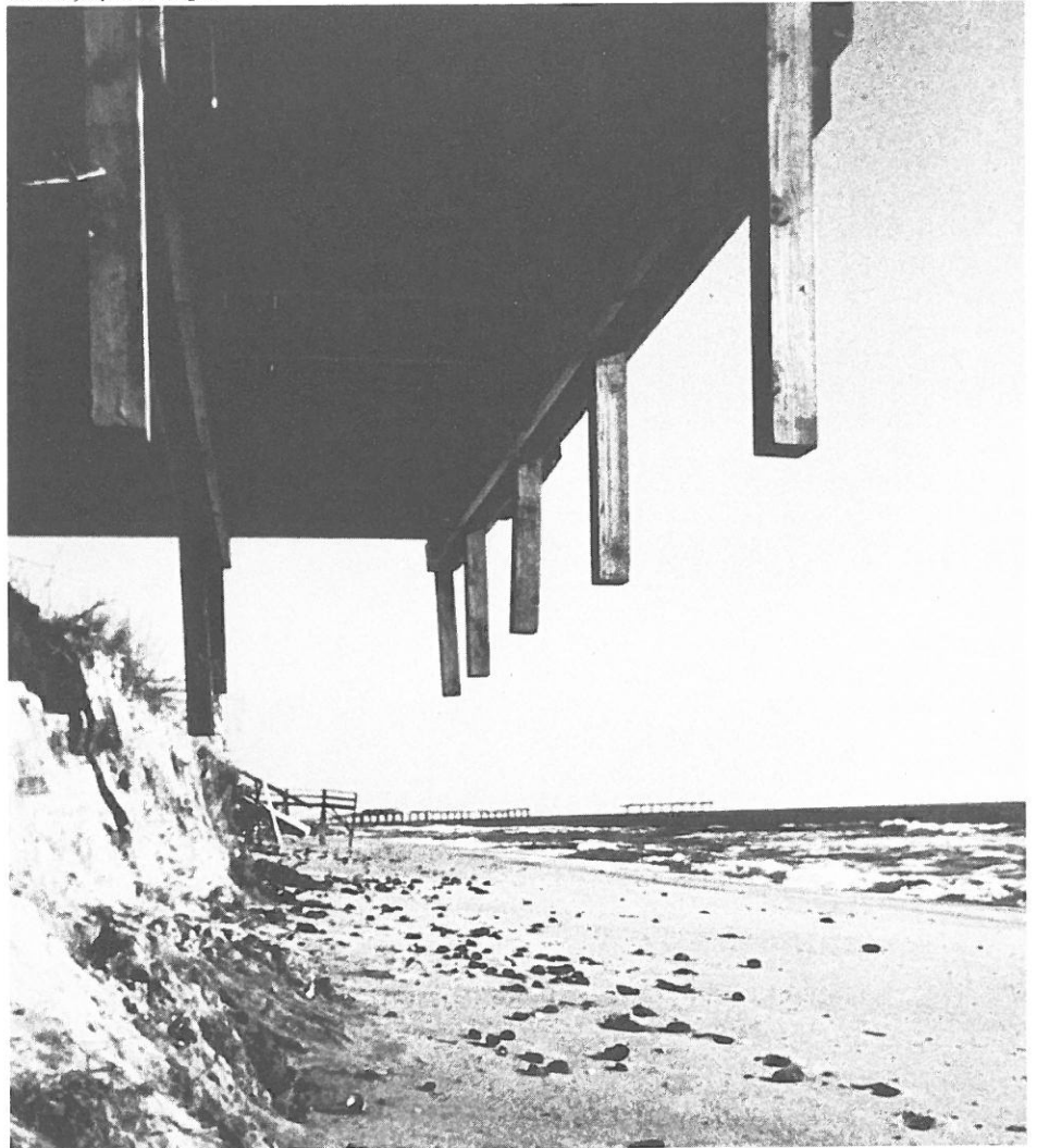
The pilings on this Carolina Beach building weren't sunk deep enough to withstand the temporary erosion caused by Hurricane David
