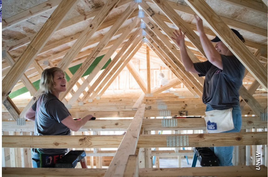
Volunteers from the UNCW Women’s Studies and Resource Center participate in Habitat for Humanity homebuilding projects that include steps to increase resilience for roofs.
