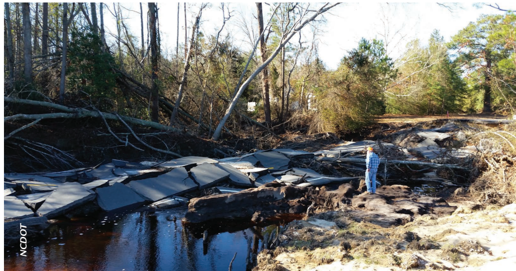
DURING AND AFTER MATTHEW, STRETCHES OF MAJOR HIGHWAYS AND INTERSTATES WERE COMPLETELY UNDER WATER, AND MANY LOCAL ROADS WERE IMPASSABLE, IMPERILING RESIDENTS AND INFLECTING HARDSHIPS.
