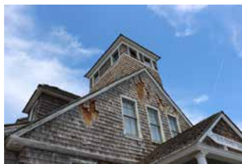
Chicamacomico Life-Saving Station needs repairs after Hurricane Arthur in July 2014.
