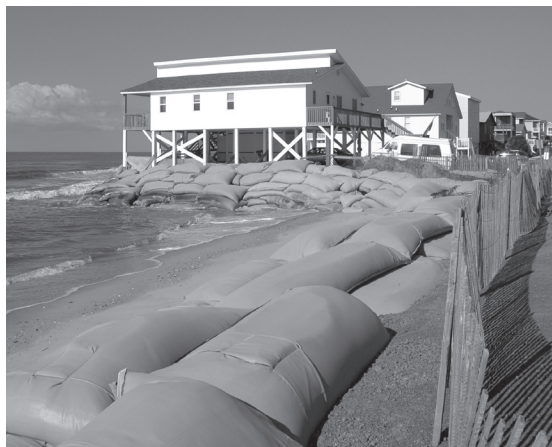
According to North Carolina law, sandbags are supposed to be a temporary fix for beachfront structures threatened by erosion. Photo: Spencer Rogers
