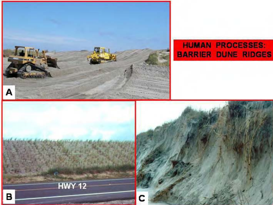
Figure 2-13. Panel A. Photo shows N.C. Department of Transportation bulldozers rebuilding a new barrier dune ridge after Hurricane Isabel in 2003. Panel B. Looking east at the newly constructed and vegetated barrier-dune ridge built to protect the post-Hurricane Dennis relocated N.C. Hwy. 12 (Figure 2-2B). Panel C. Photograph of the ocean side of a recently constructed barrier dune ridge that shows severe erosion and scarping of the barrier dune ridge that is totally out of equilibrium with the ocean dynamics. Photographs are by S. Riggs.
